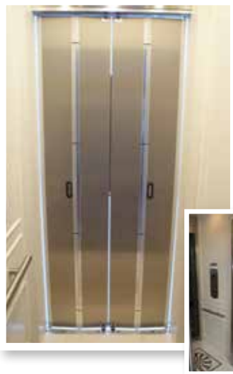
Automatic Bifold Gate View from inside elevator
