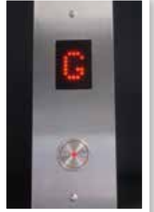
Located in hallway. DPI displays the floor your elevator is servicing
