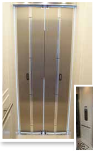
Automatic Bifold Gate View from inside elevator
