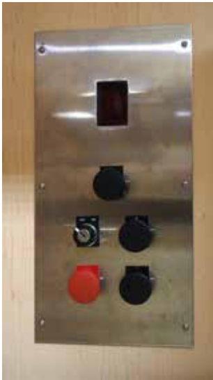
Car Operating Panel located inside the cab
